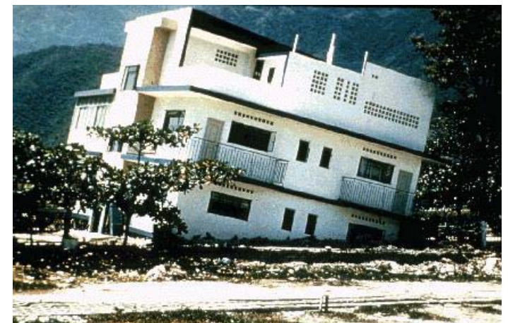
The 1967 earthquake in Caracas, Venezuela killed 240 and caused $50 million in property damage. Here, a building tips over due to soil liquefaction and resulting foundation failure.
