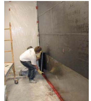
Workers retrofit Verizon Southern California central office, one of some 2,000 buildings that have been protected with UCSD's carbon overlays.
